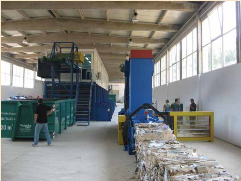
Photo 3.3 Recycling Plant in Bosnia and Herzegovina
