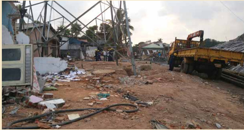
Photo 7.6 Recovery Efforts after Meethotamulla Dumpsite Collapse from Heavy Rains in Colombo, Sri Lanka
