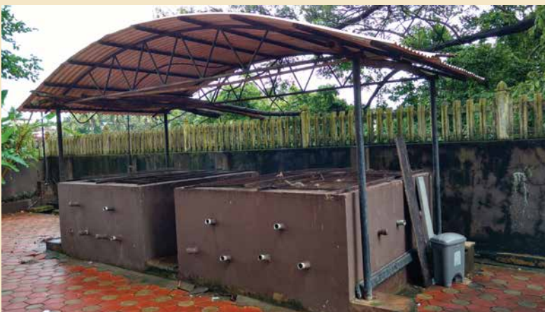
Photo 7.8c Decentralized Composting Units in Panaji, India
